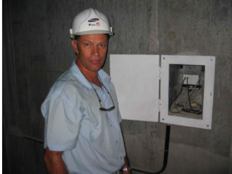
Installation of NIVEL200 in the Burj Dubai - world tallest building - by Doug Hayes
